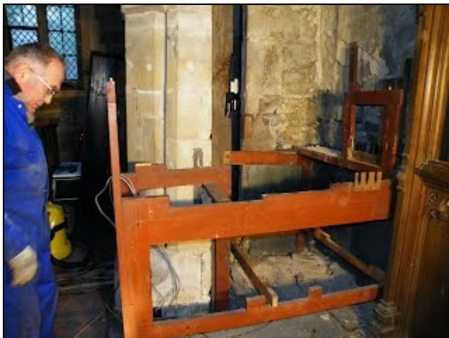
The frame of the Ansty organ reveals that it was built around an old door arch, which possibly led to a medieval rood loft stairs. Stephen Taylor surveys the remains of the organ. (Picture: Richard Young)
